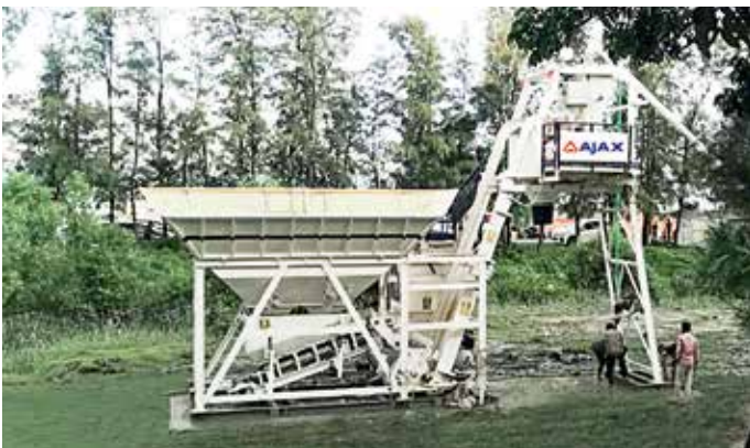
AJAX Batching Plant operating in Chittagong.
